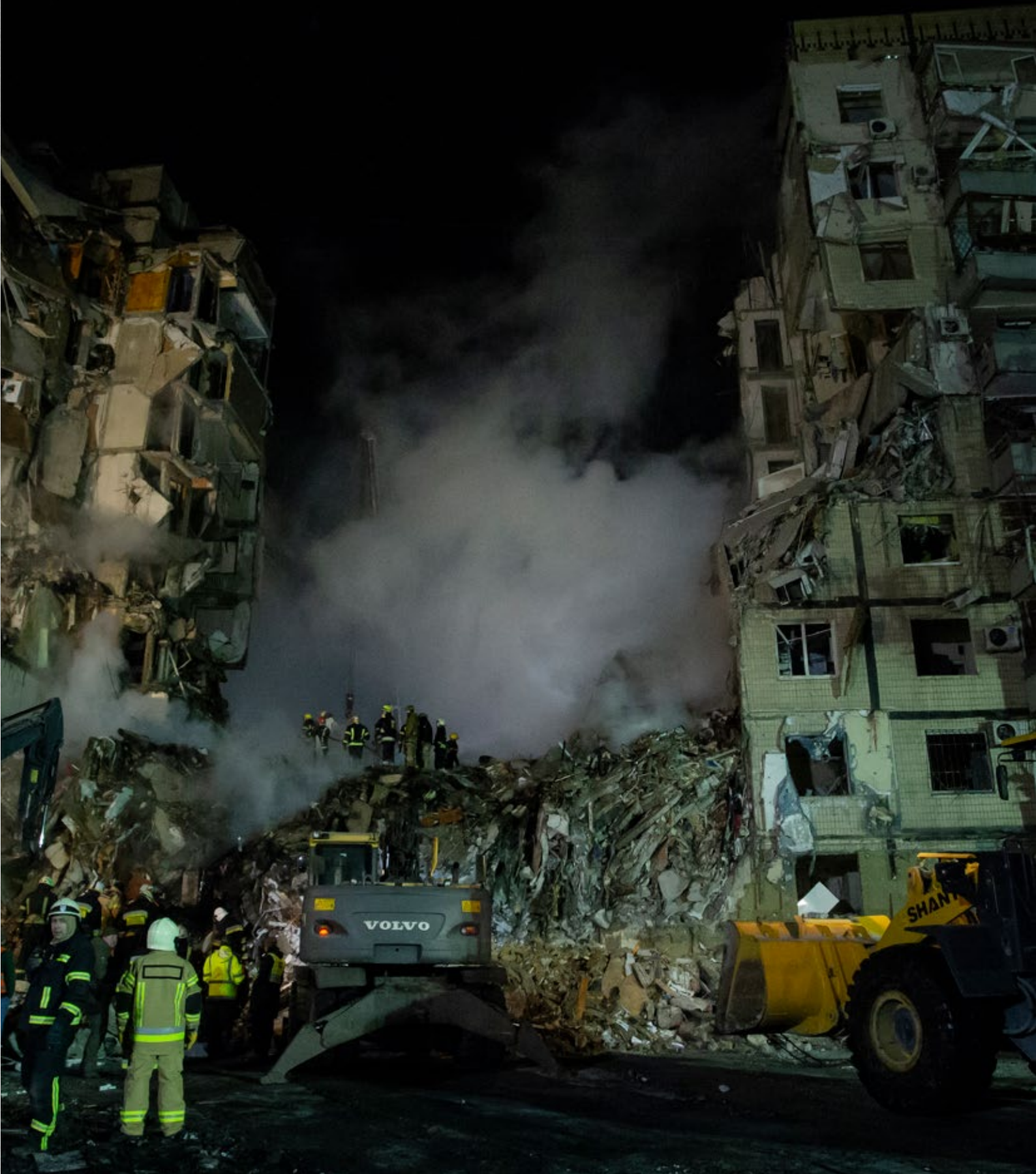
On 15 January 2023 in Dnipro, Ukraine, firefighters stand near a dump truck as colleagues carry out search and rescue operations at a residential building hit the previous day by a Kh-22 cruise missile that destroyed one section of the nine-storey building and killed 21 people. — © 2023 Global Images Ukraine — Yan Dobronosov
